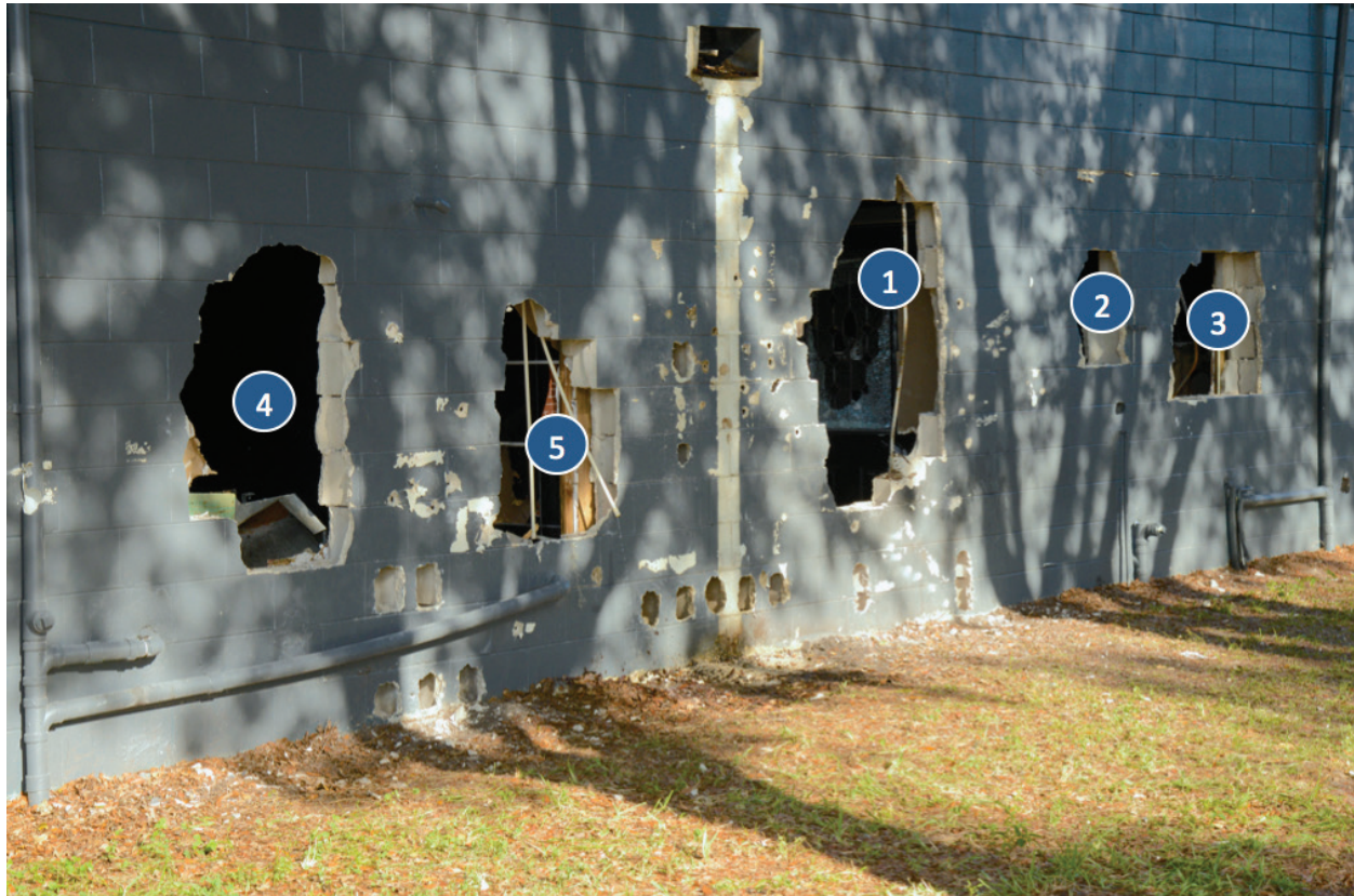
Figure 6. Breaches of Pulse nightclub exterior wall
